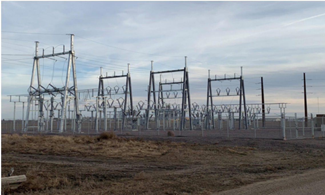
Figure 32: Aberdeen A-Tap Switchyard
